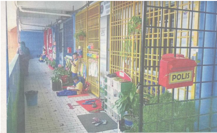
Grilles are installed at the kindergarten in the Seri Selangor commercial complex.
