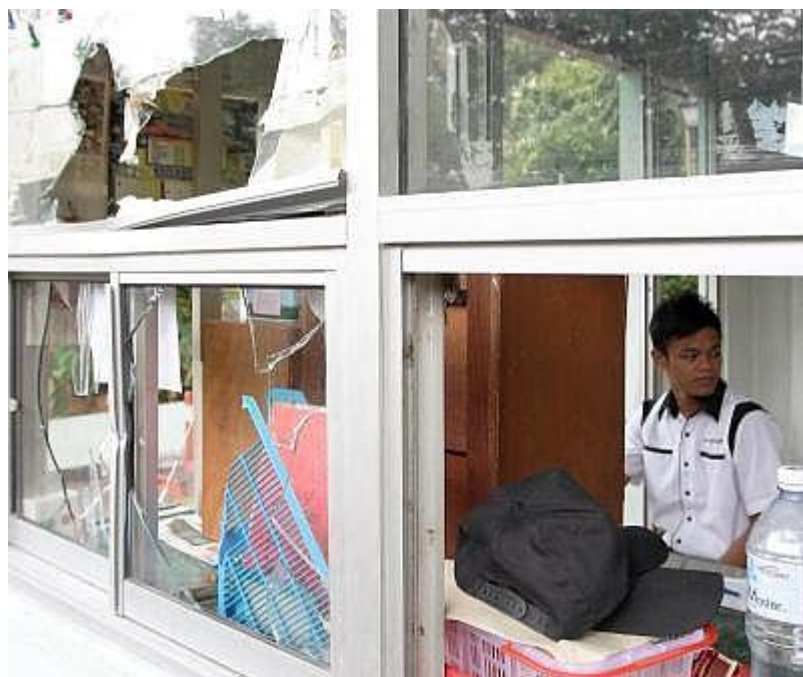
Damaged: The security guard post is not spared from the mob attack.
